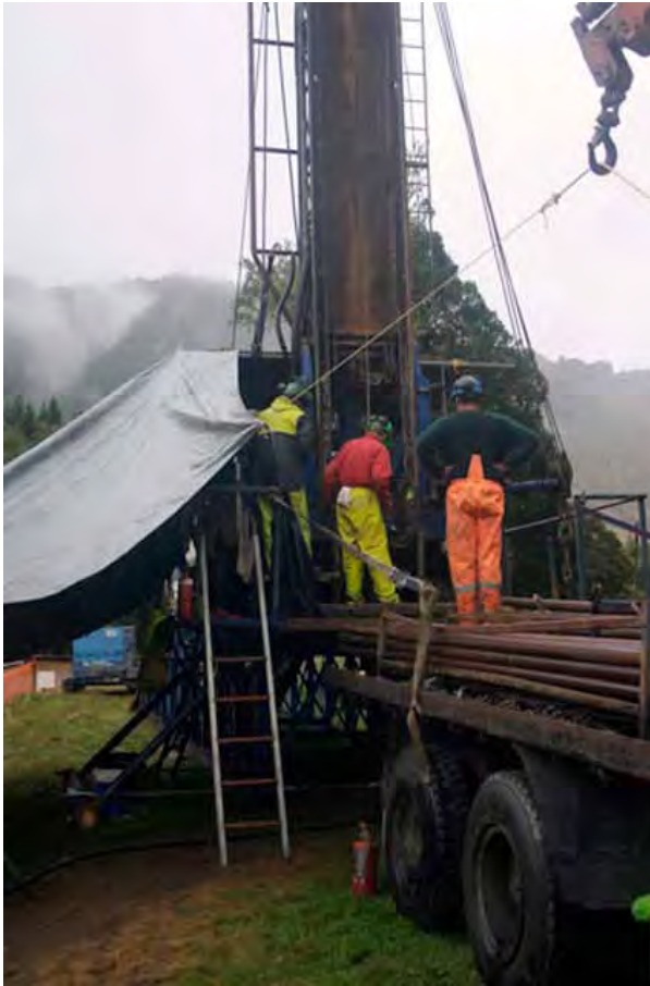
Figure 4. Failing rig supplied by CW Drilling of Motueka, A single stage BOP/diverter Owned by Western Exploration was employed and fitted beneath the Sub.
